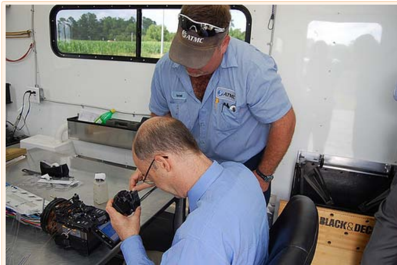
Rural Development Utilities Administrator Jonathan Adelstein receives lesson in fiber splicing. Photo credit: USDA employee Delane Johnson.
